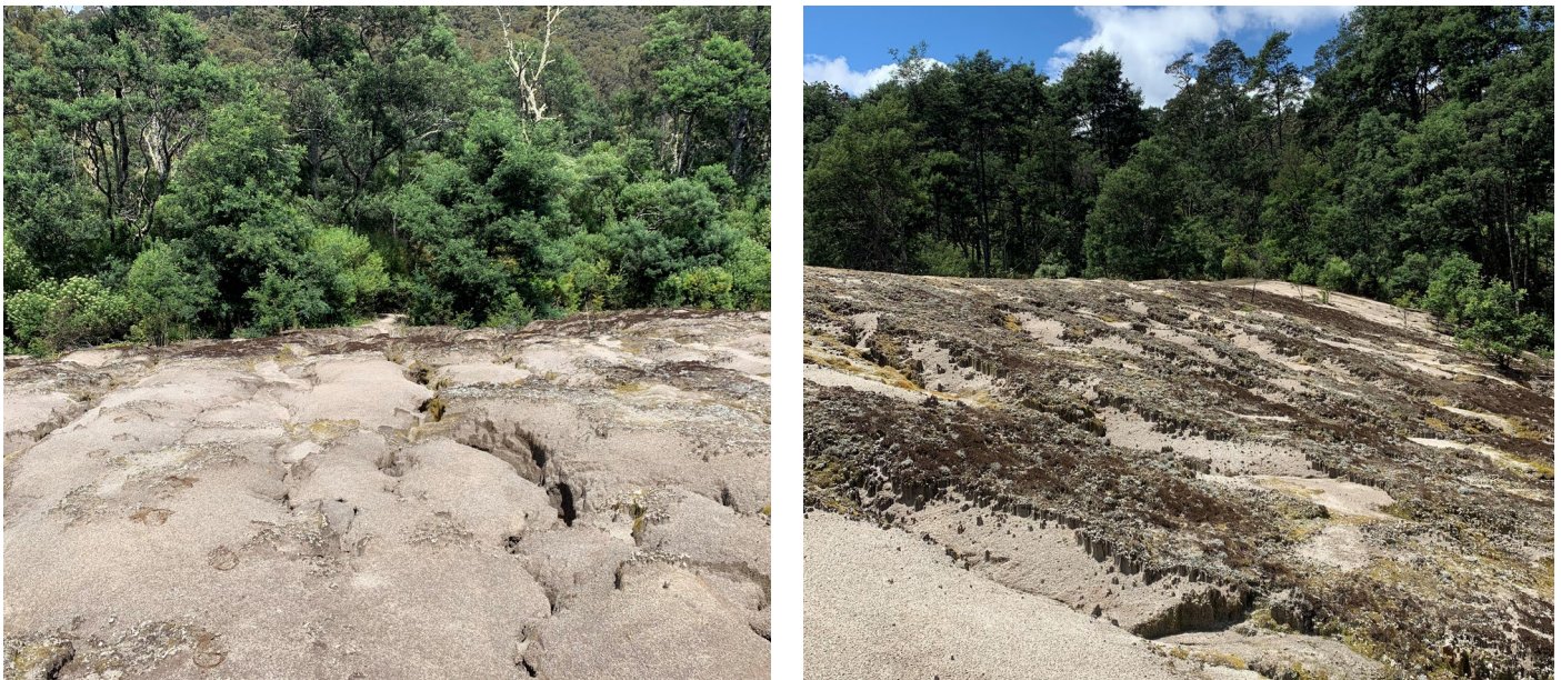
Figure 2. Erosion mitigation required on the Anchor dam wall (October 2024).
