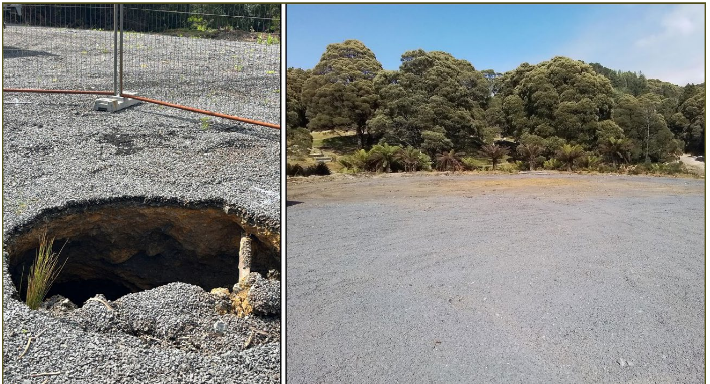
Figure 10. Sinkhole (left) and completed remediation (right), Zeehan Cemetery, March 2025.
