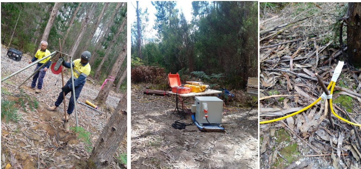
Figure 3: Khumsup survey crew in action dummifying the hole, and several shorts of the equipment
